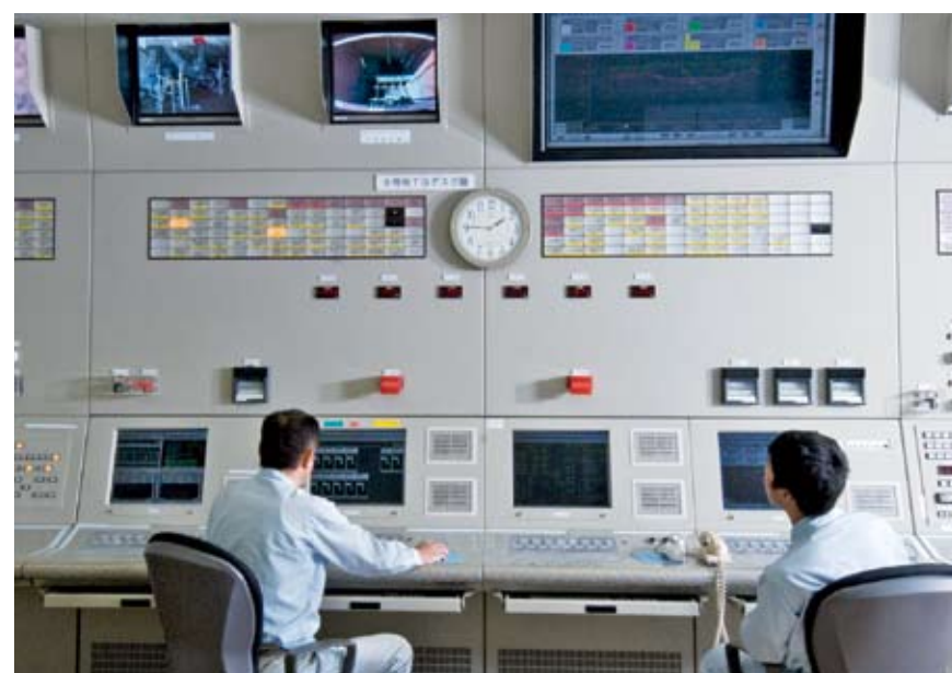
Tosoh is the Japanese leader in the in-house generation of electricity, and it optimizes its generating operations with state-of-the-art control systems.
