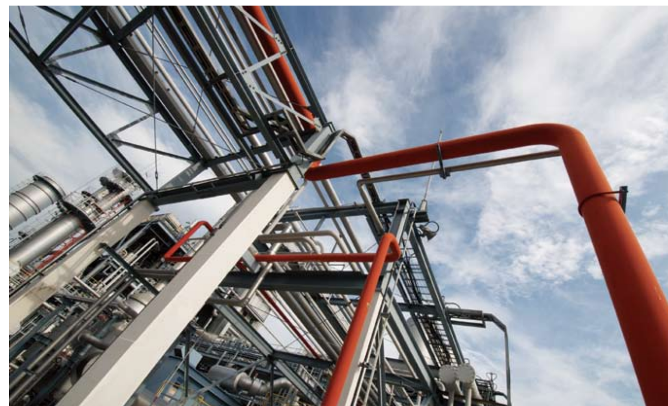
Newly expanded production facilities for carbon monoxide are another link in Tosoh's vinyl isocyanate chain.
